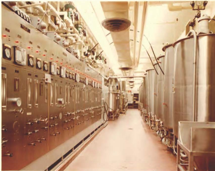
FIGURE 8 - Chemical Mix Room
