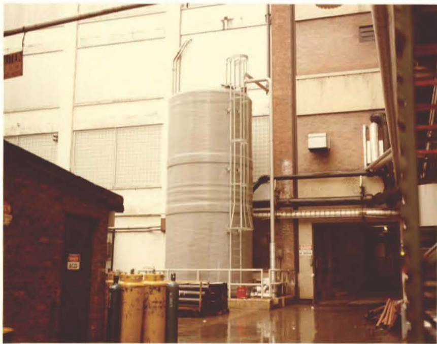
FIGURE 46 - Effluent Collection Tank
