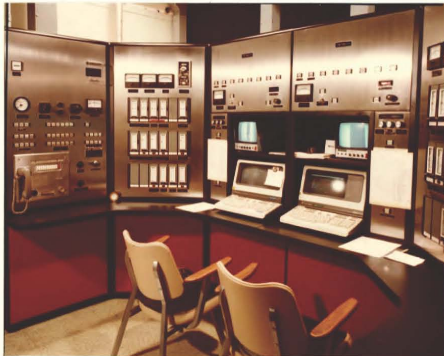
FIGURE 25 - Ontario Control/Monitor Area
